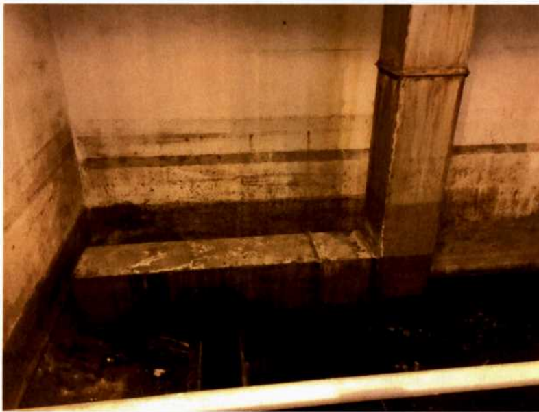
Figure 16: Headworks Chamber Exhaust Hood and Duct
