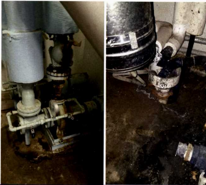
Figure 17: Boiler Circulation Pumps and Drain
