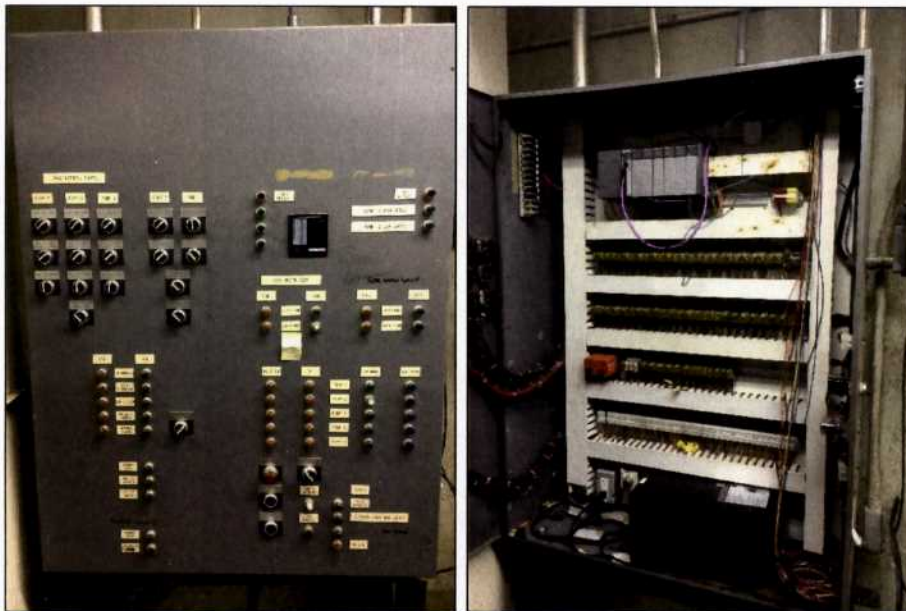
Figure 22: Pump Control System Panel
