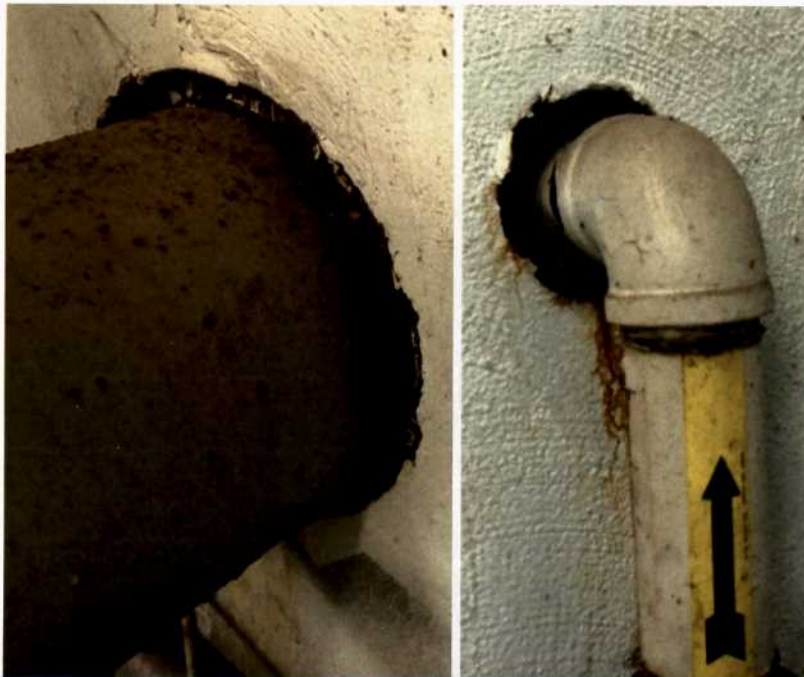
Figure 11: Drywell Pipe Penetration Seals
