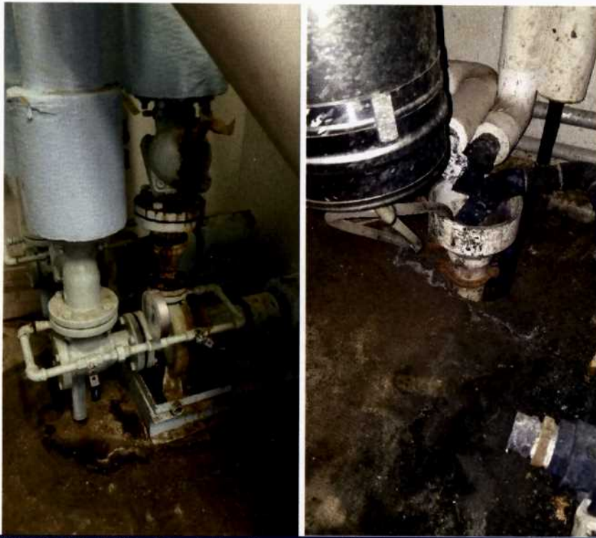
Figure 17: Boiler Circulation Pumps and Drain
