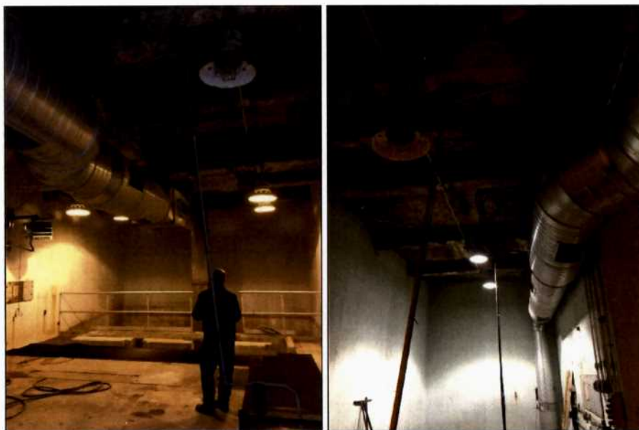
Figure 19: Headworks Chamber Original Lighting (left) and new LED lighting (right)
