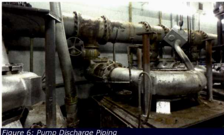
Figure 6: Pump Discharge Piping
