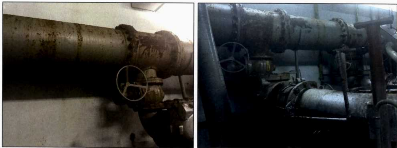
Figures 1 and 2: Exterior of the Lift Station Header Piping
