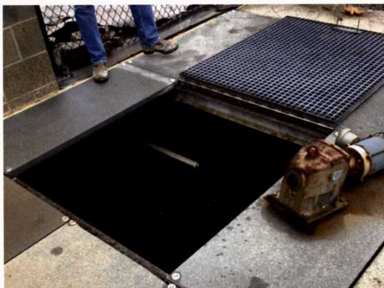
Figure 8: Wet Well Access Panels
