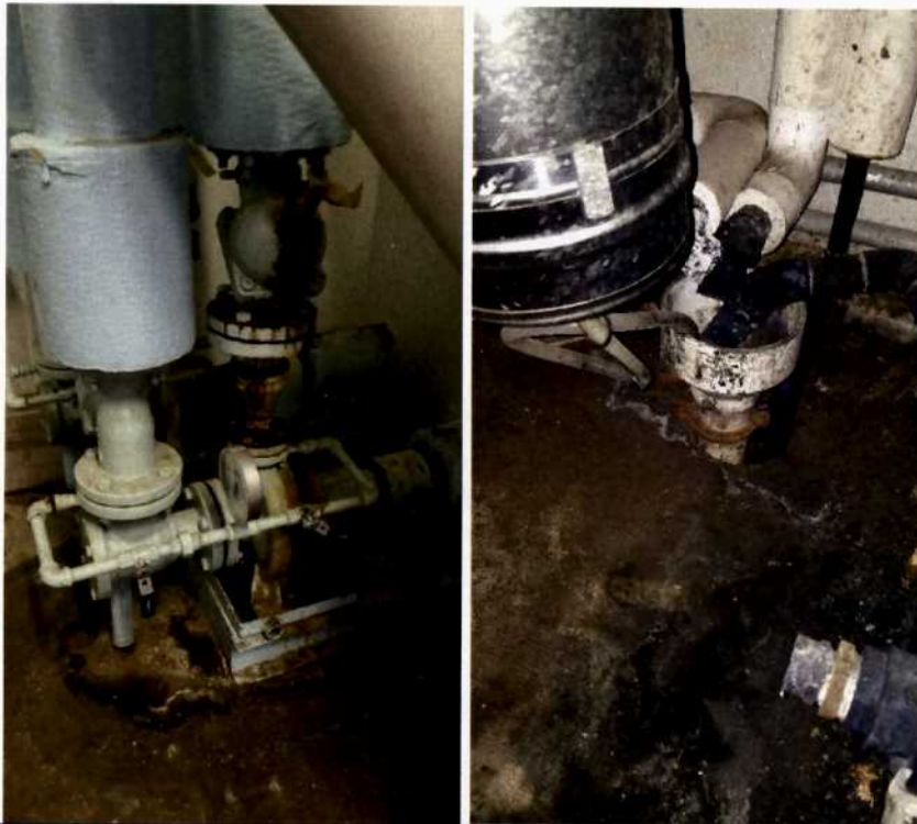
Figure 17: Boiler Circulation Pumps and Drain
