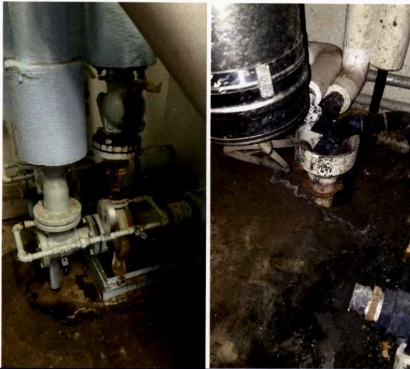
Figure 17: Boiler Circulation Pumps and Drain
