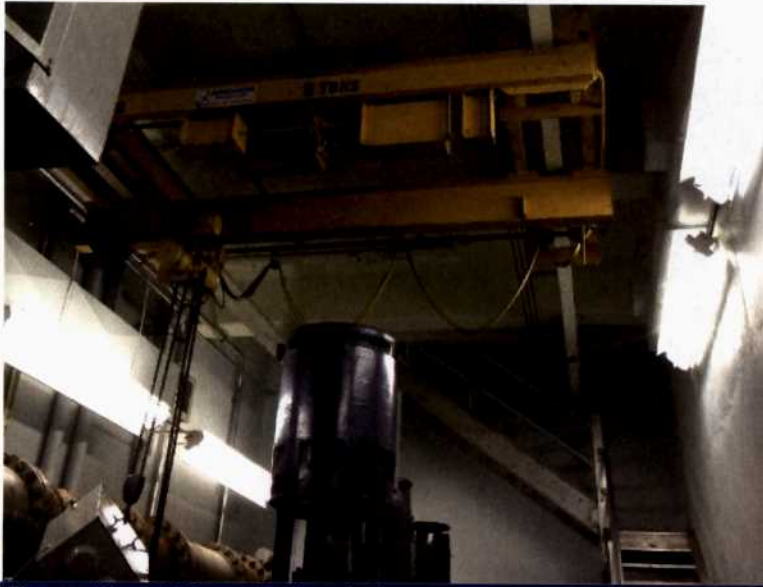
Figure 10: Existing Overhead Crane
