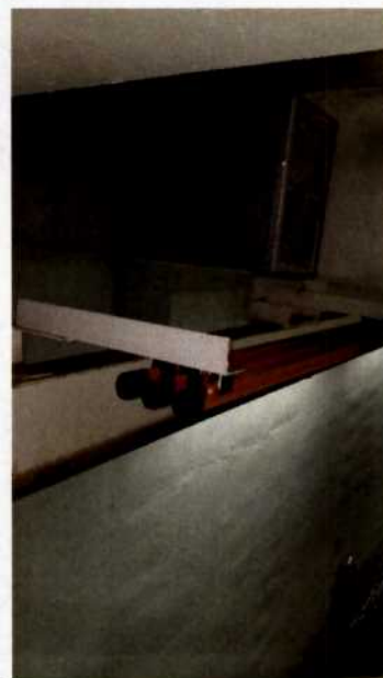
Figure 20: Electric Hoist Bus Bar near stair handrail
