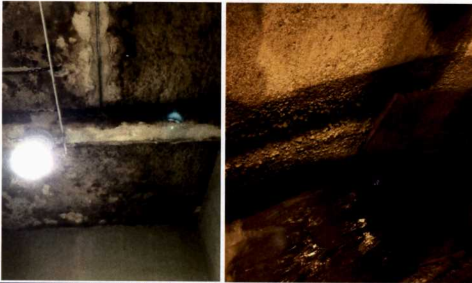
Figure 14: Headworks Chamber Ceiling and Channel concrete spalling
