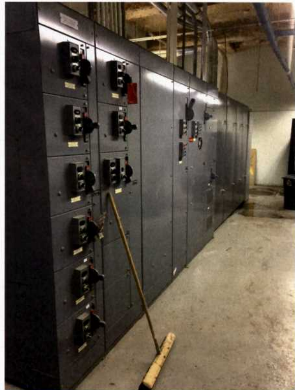
Figure 18: Existing Motor Control Center
