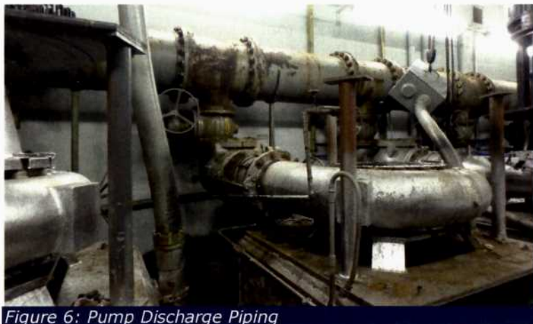
Figure 6: Pump Discharge Piping
