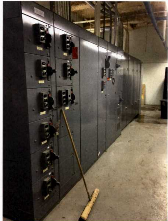
Figure 18: Existing Motor Control Center
