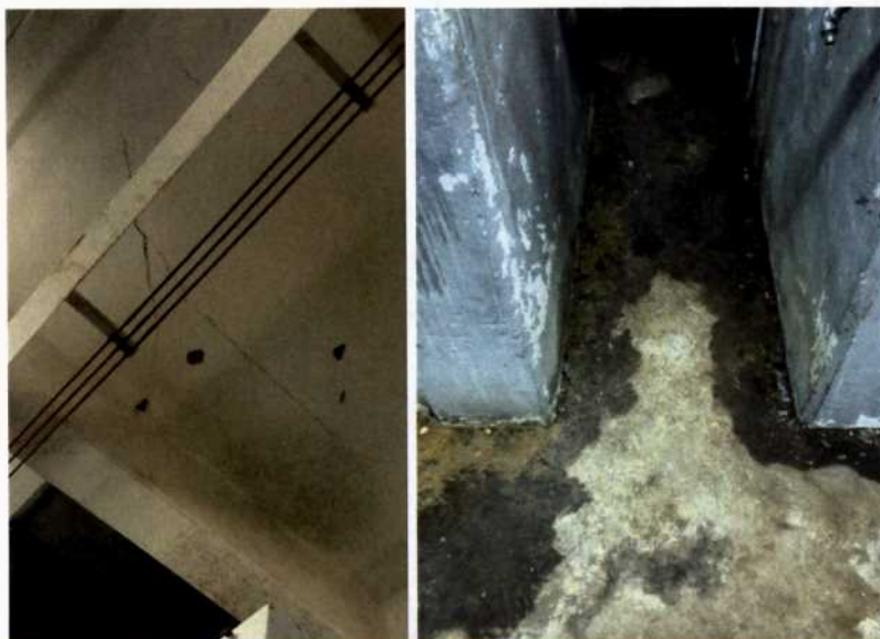
Figure 12: Pump Room Ceiling Cracking and Floor Slab
