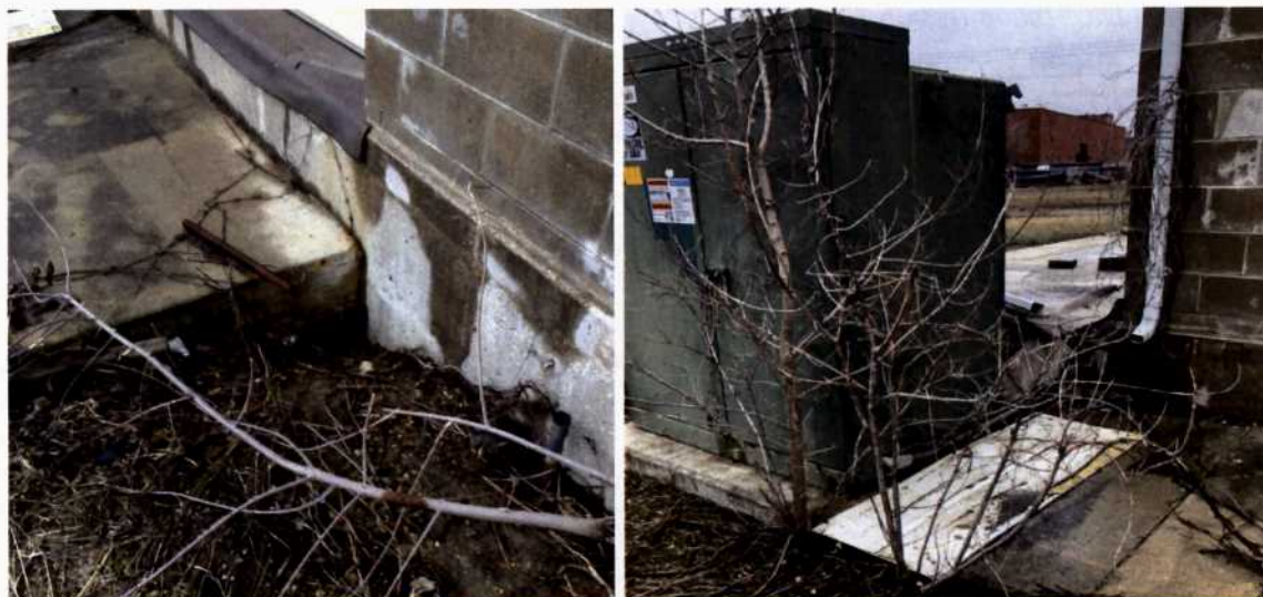
Figure 2: Animal Burrows, downspouts, and vegetation around lift station exterior
