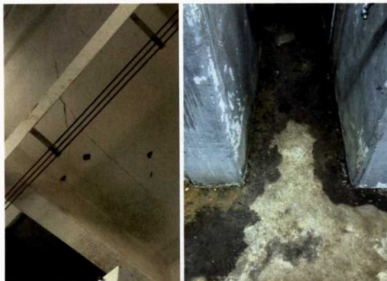
Figure 12: Pump Room Ceiling Cracking and Floor Slab
