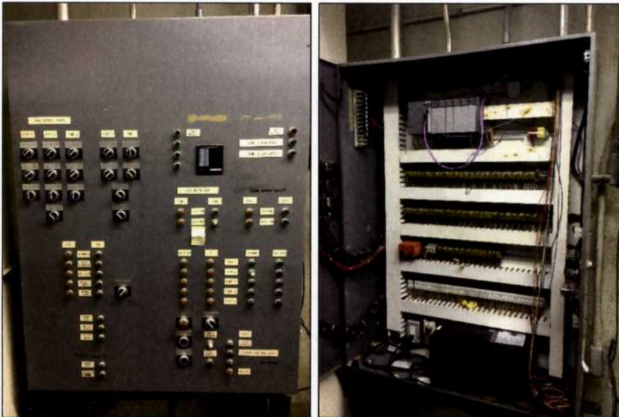
Figure 22: Pump Control System Panel
