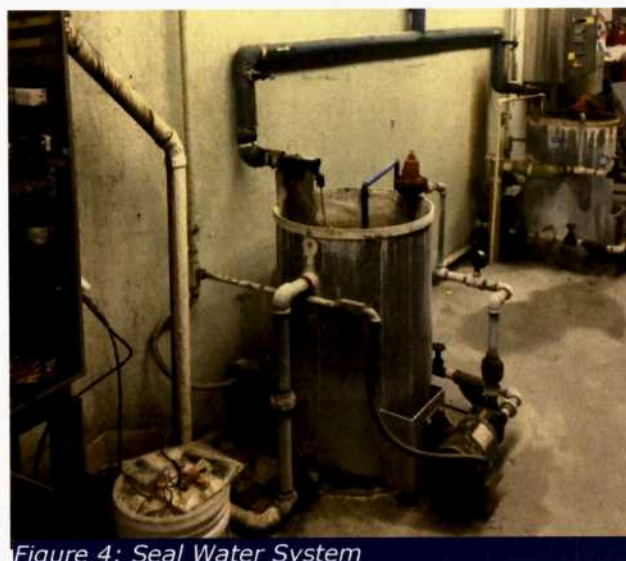
Figure 4: Seal Water System
