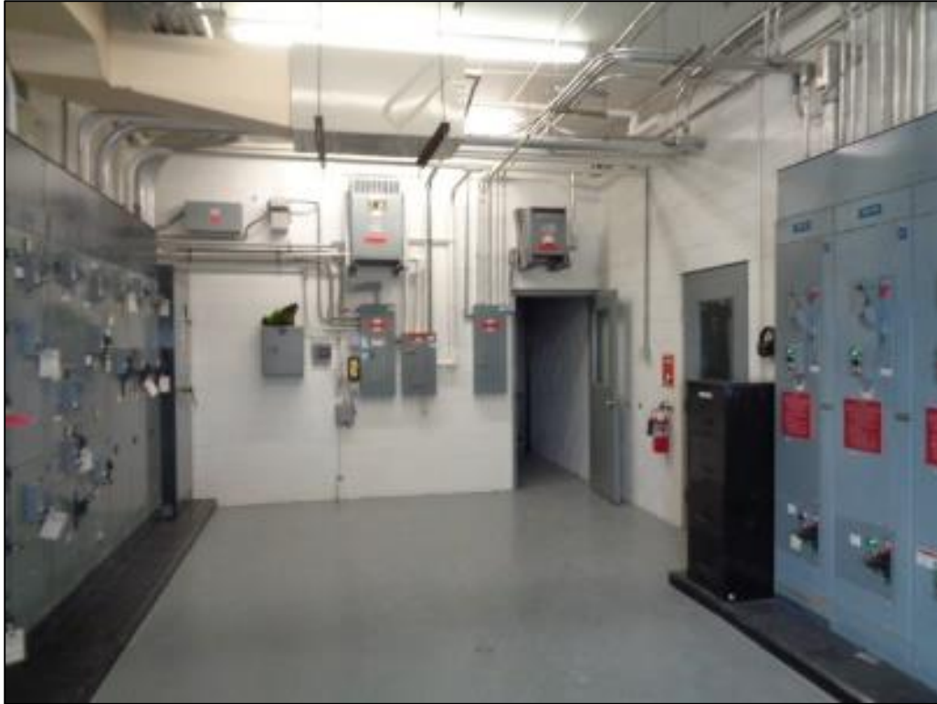
Electrical For Concrete Pits
