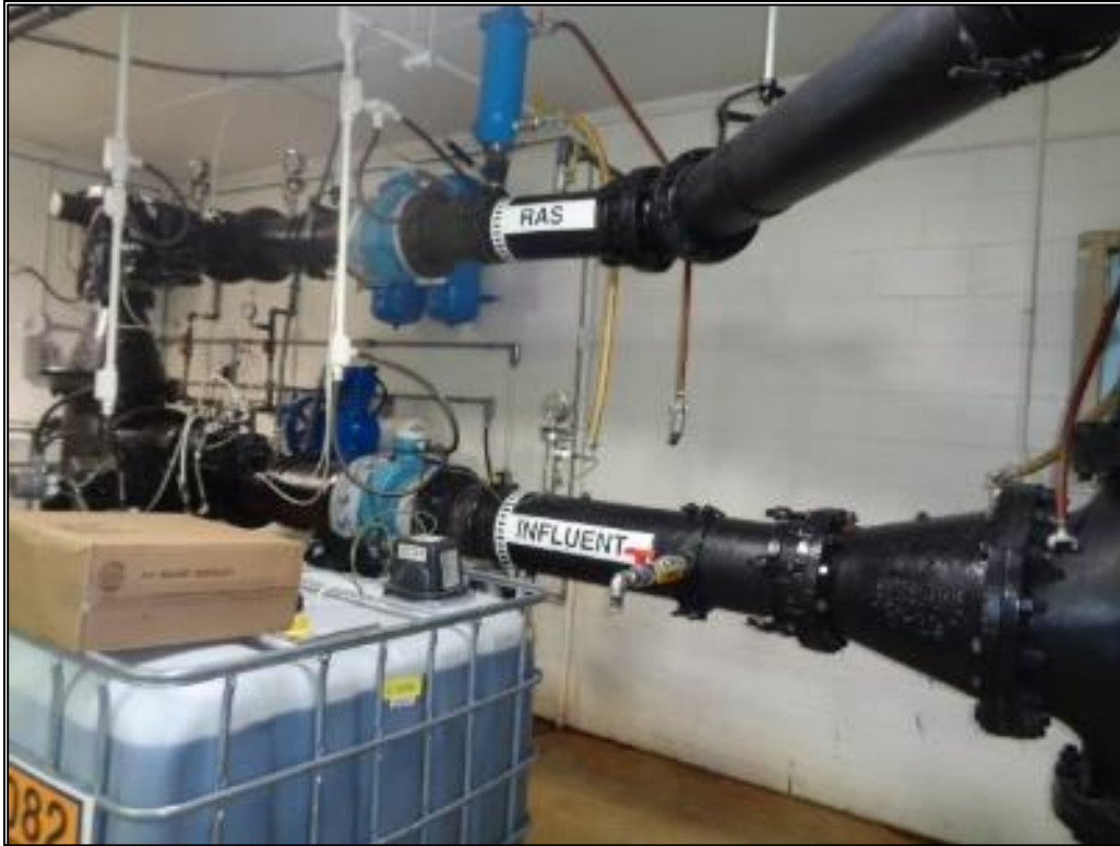
Pump Area For Concrete Pits
