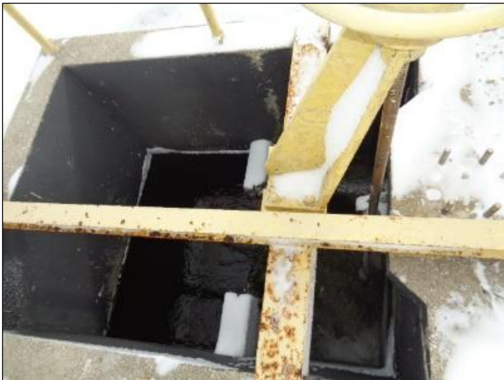
Clean Water Discharge
