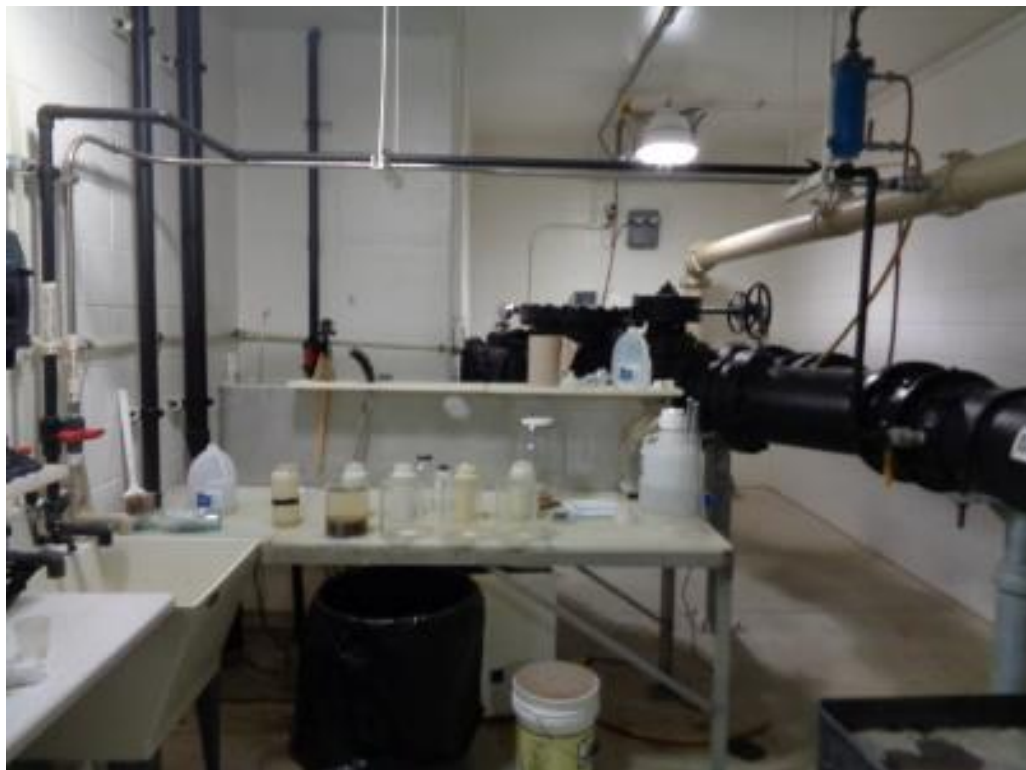
Pump & Lab Area For Concrete Pits
