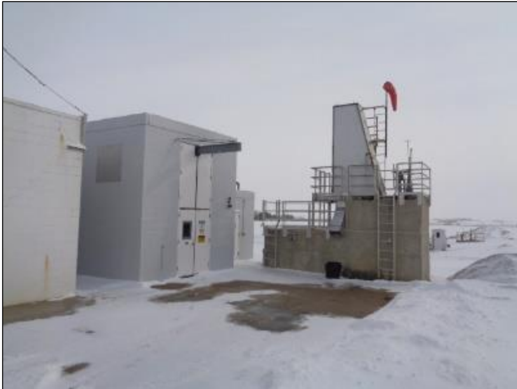
Exterior – Chlorine Injection Area
